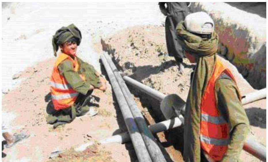
Workers in Tirin Kot excavate to identify damaged and broken components of the water supply system; providing safe drinking water is a nationwide challenge.
