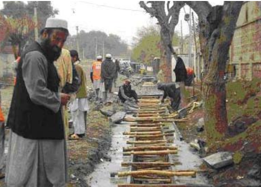
Workers in Jalalabad make improvements in a ditch that is part of the city's sewage system.
