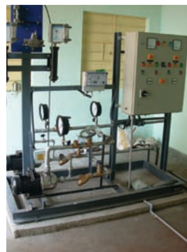
Chlorinators help improve water quality
