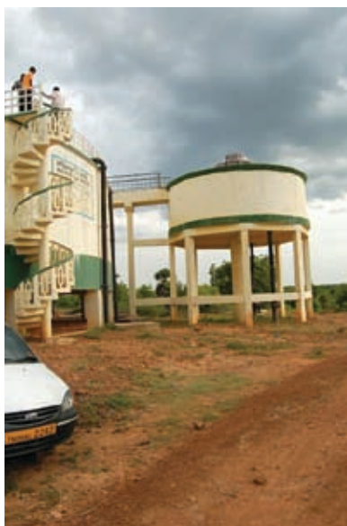
Overhead tanks are part of the water distribution system.
