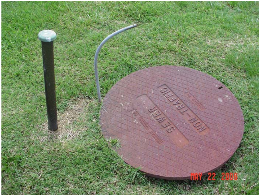
Figure 3.3 – Valve Pit Lid and External Breather
