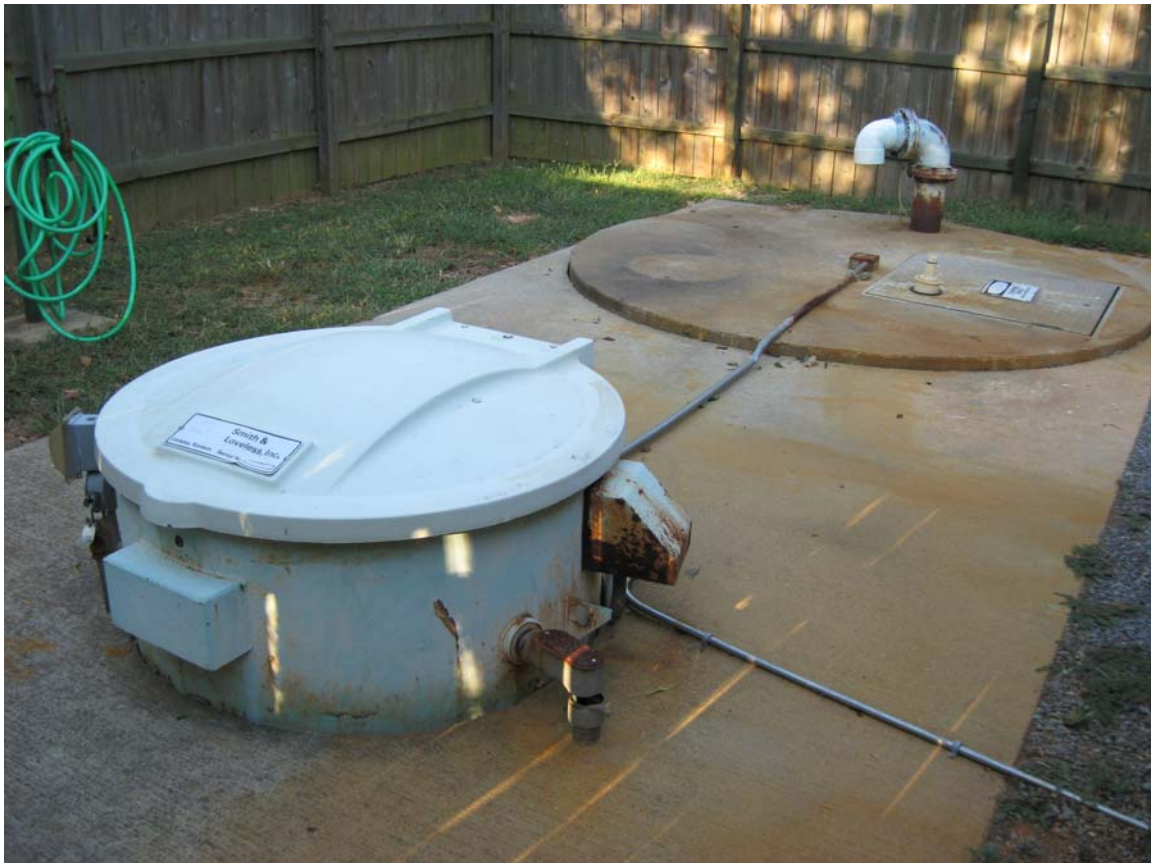
Figure 4.11 – Tyree Springs Lift Station
