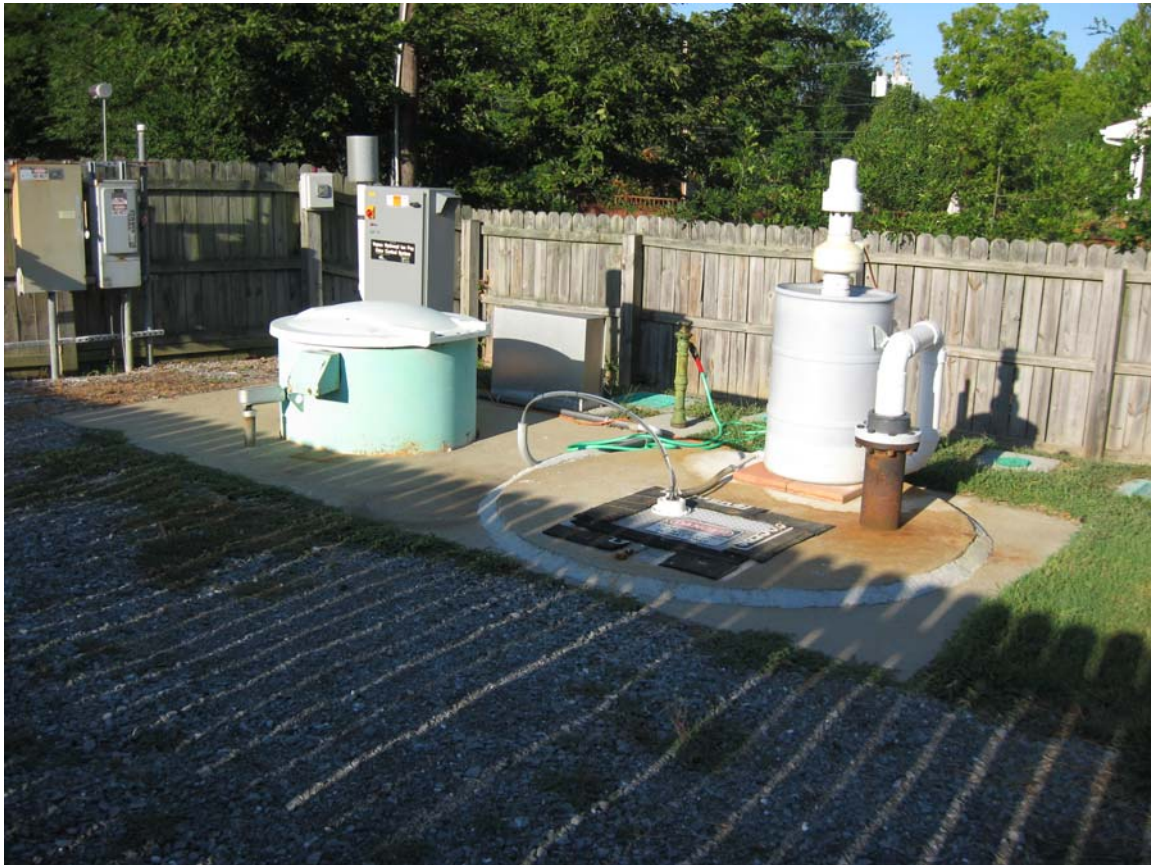
Figure 4.13 – South Palmer's Chapel Lift Station
