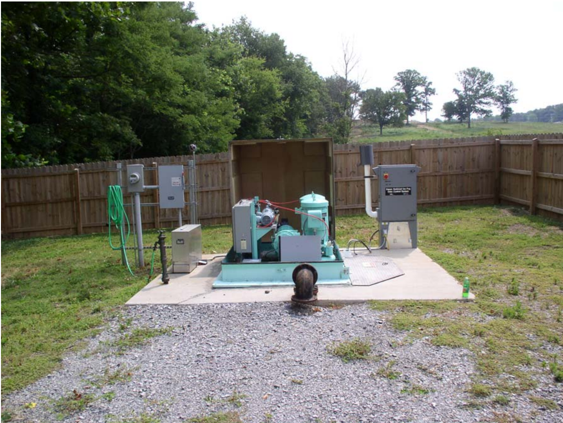
Figure 4.15 – Union Road Lift Station
