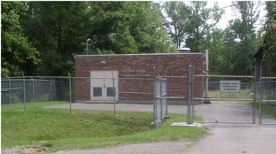
Figure 4.7 – Calista Road Vacuum Pumping Station
