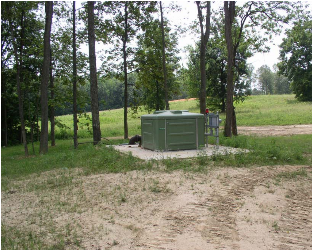
Figure 4.17 – Cambria Lift Station
