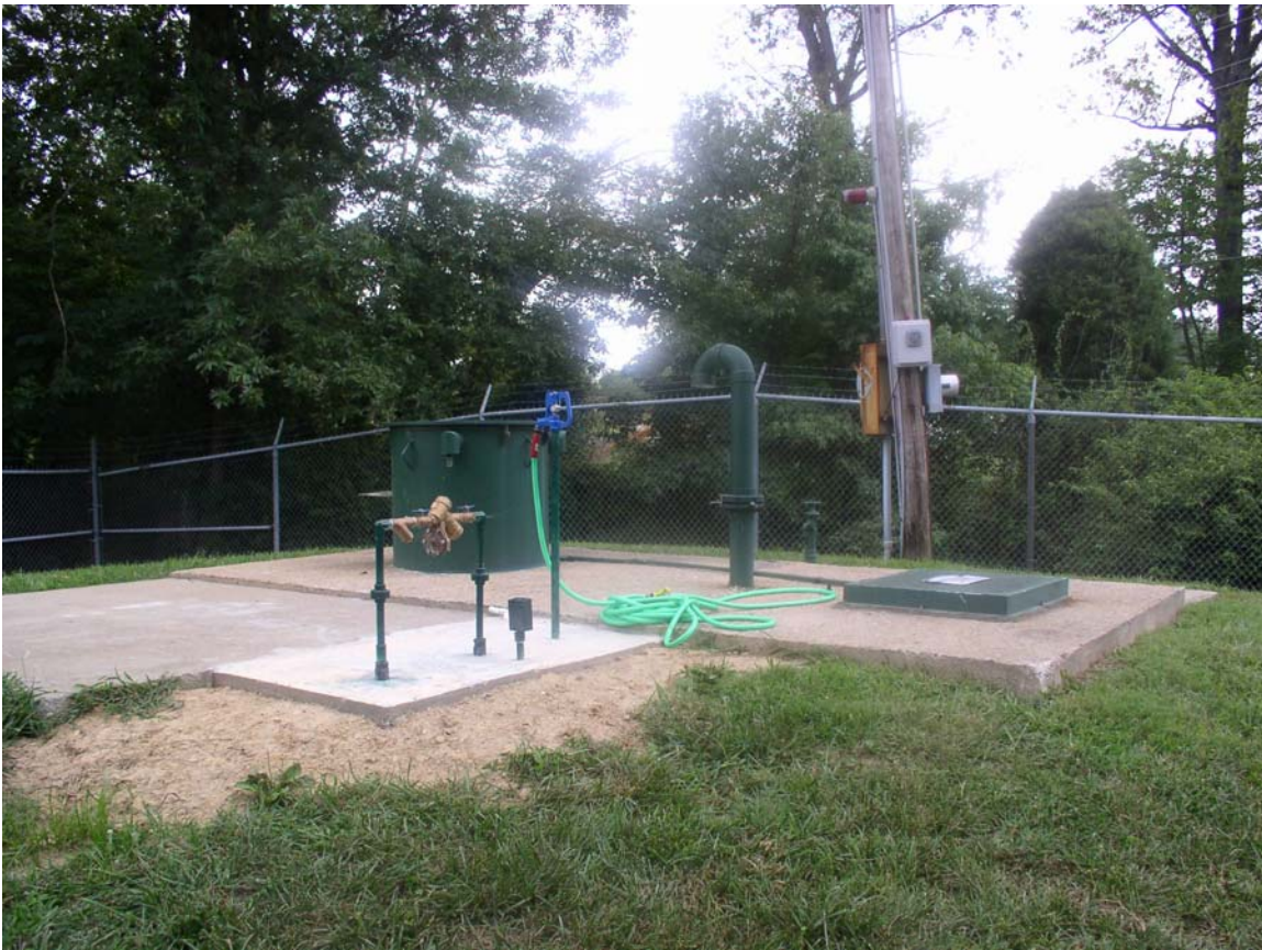
Figure 4.19 – Meadowlark Lift Station
