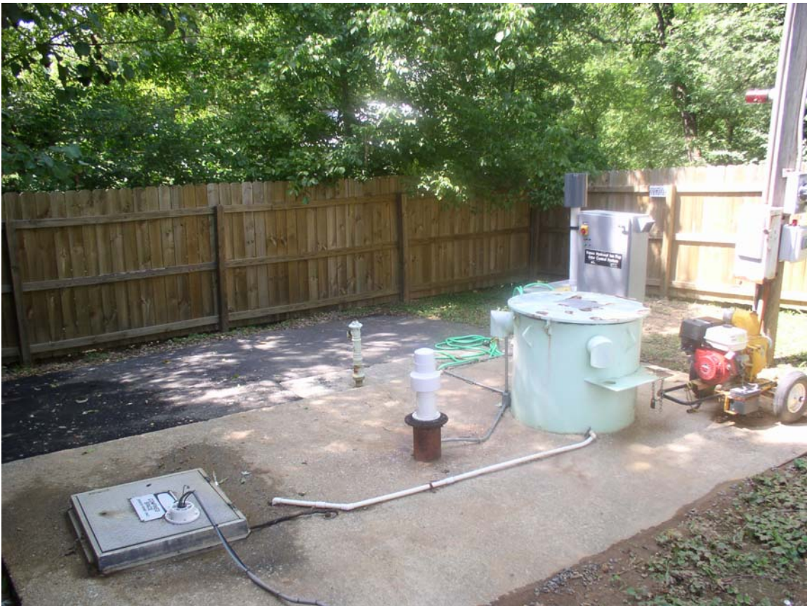
Figure 4.9 – Wilkinson Lane Lift Station
