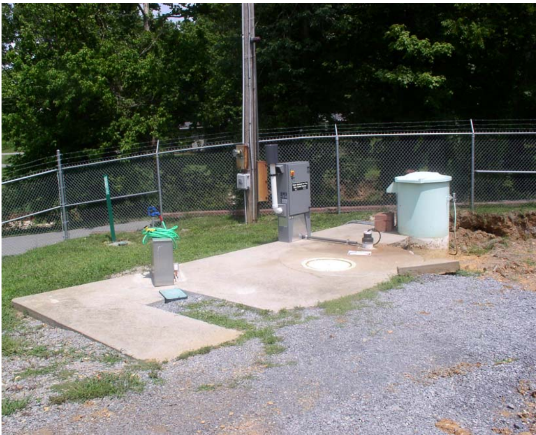
Figure 4.5 – Portland Road Lift Station
