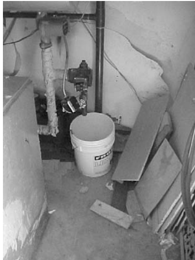
A 37-year-old DPW worker was electrocuted in this boiler room while attempting to read a water meter.
