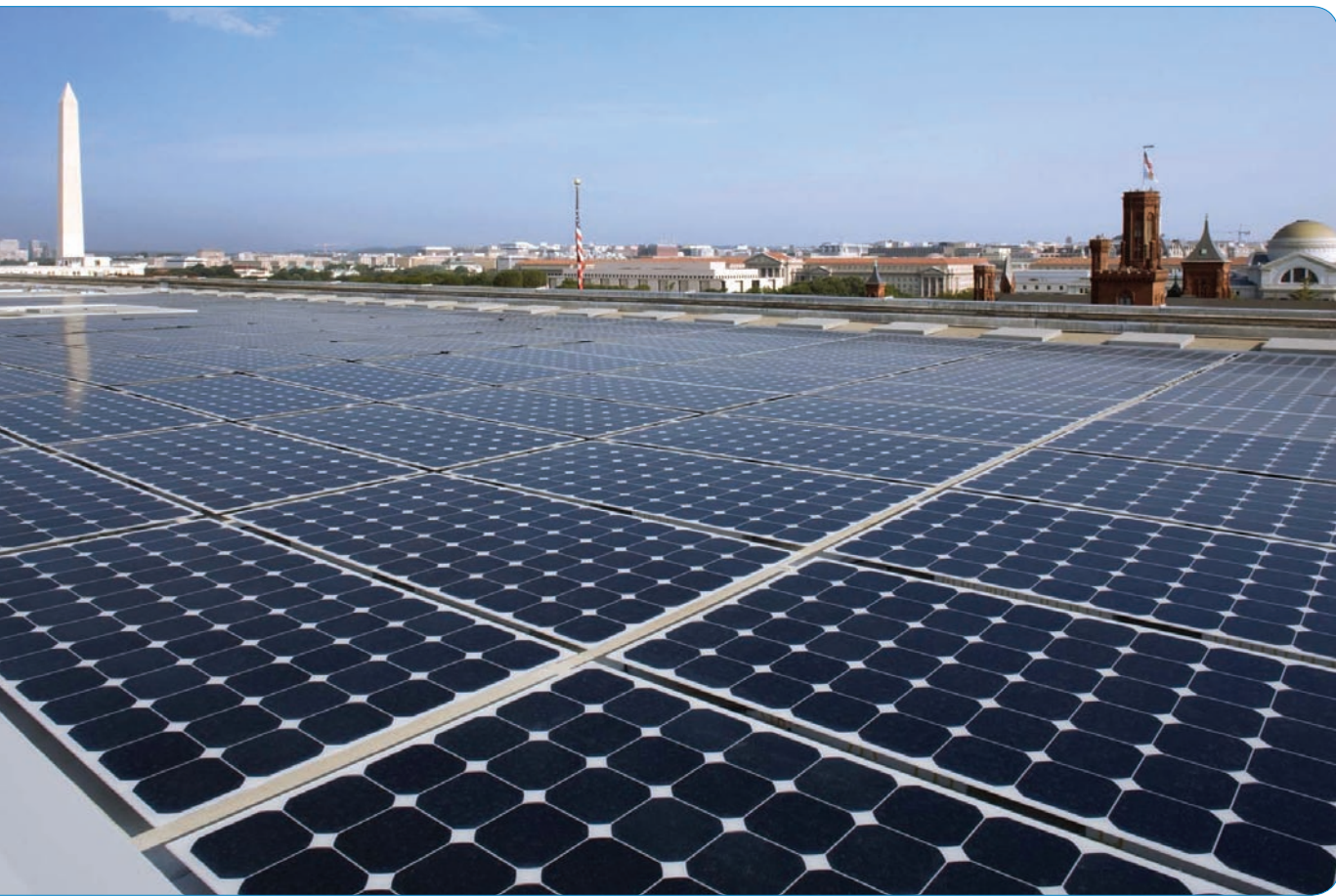
205 kW PV system installed on the U.S. Department of Energy Forrester Building in Washington, D.C. (Photo credit: SunPower Corporation)
