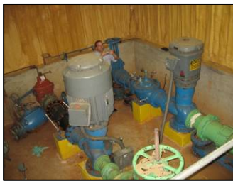
The South Buncombe Pump Station exterior and two of its three pumps
