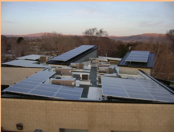
Roof view of Larry D. Johnson Community Center Photovoltaic Project
