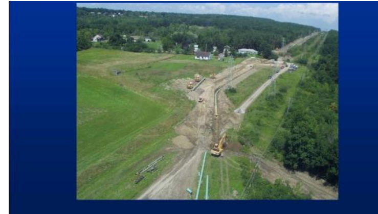
NATURAL GAS SERVICE
