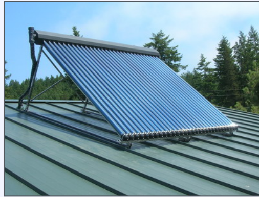
Solar Hot Water
