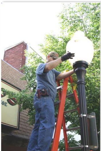
Decorative lighting in downtown Lawrence, KS was replaced with LEDs to improve lighting quality and cut energy by 30%.
