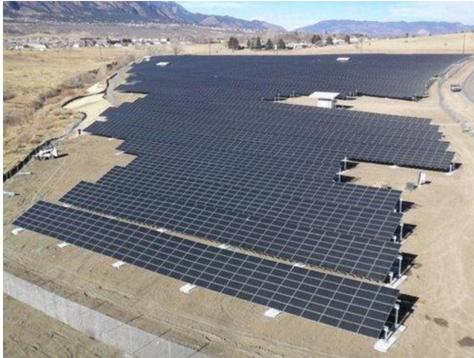
Source: NREL PIX 17394
