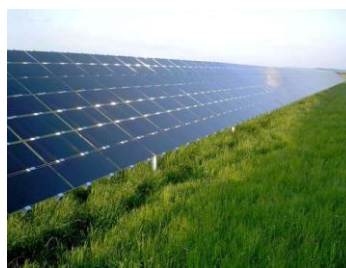
Source: NREL PIX 14726
