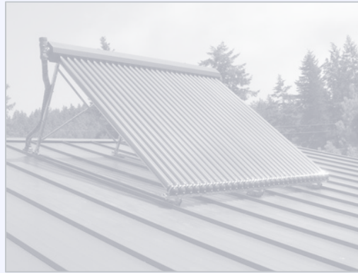
Solar Hot Water
