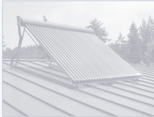
Solar Hot Water
