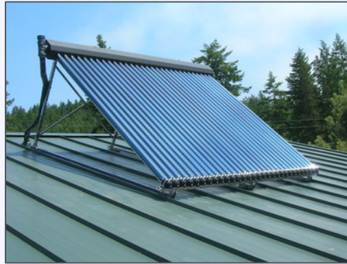
Solar Hot Water
