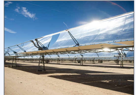
Concentrated Solar Power
