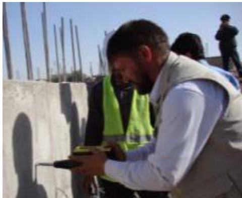
Eng. Nadir using the digital hammer to test the quality of concrete used on a municipal construction project
