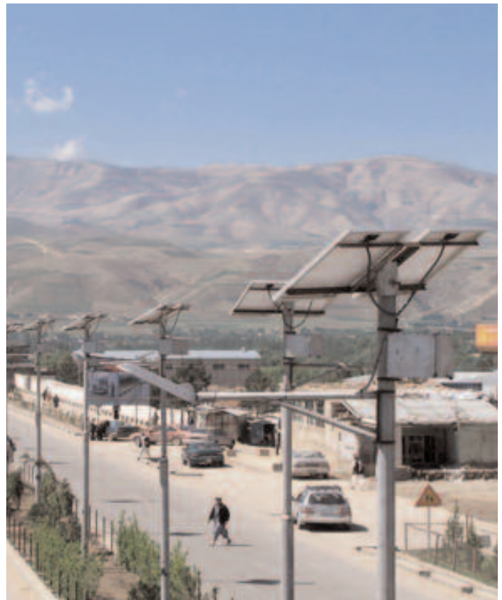
The solar streetlights in the city of Faizabad, located 600 kms from Kabul, were procured and installed under the USAID-funded Afghan Clean Energy Project (ACEP). The city is not connected to the national power grid. Credit: Abdul Raso.
