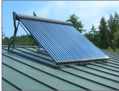
Solar Hot Water
