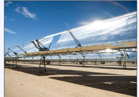
Concentrated Solar Power
