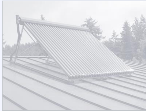
Solar Hot Water
