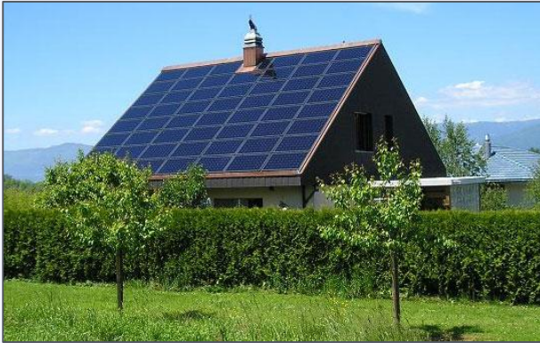
Solar Photovoltaic (PV)
