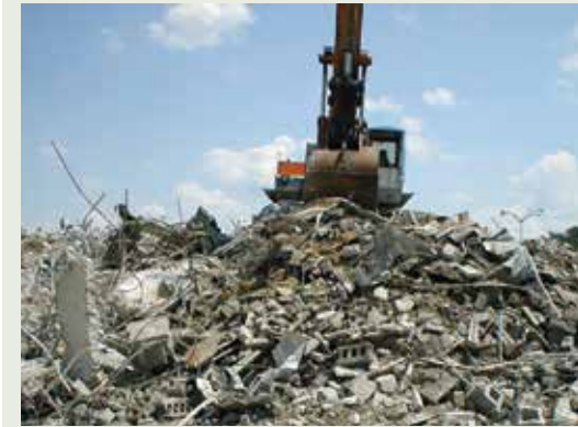
The demolition and brownfield remediation of the Akron-Middlebury Grocery in Akron, Ohio.
