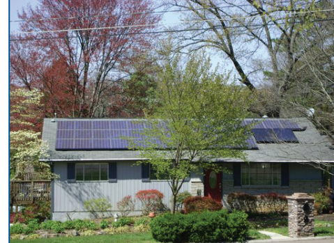
A PV System installed on a residence. (Photo credit: Courtesy of DOE/NREL)
