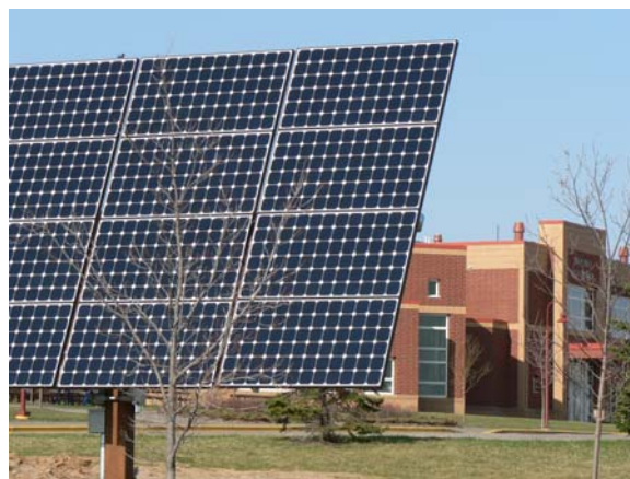
Figure 2: The 3.7 kW PV system installed at the River Falls High School (photo courtesy of RFMU).
