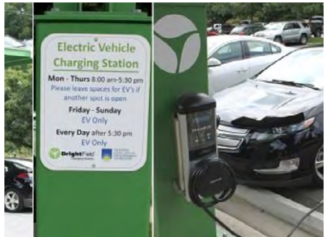
City of Asheville Electric Vehicle Charging Stations
