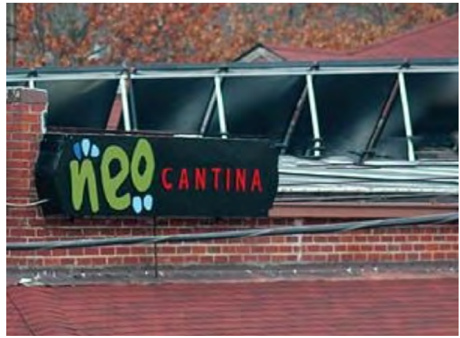
Solar panels on Neo Cantina 13
