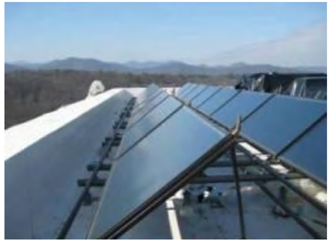
Solar panels on the roof of the Hilton Asheville Biltmore Park.
