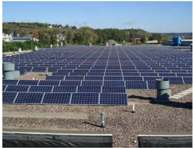
The City of Dubuque partnered with a local solar company to create one of the state's largest solar installations. More than eight hundred panels are situated atop the city's Municipal Services Center. Photo courtesy of City of Dubuque.
