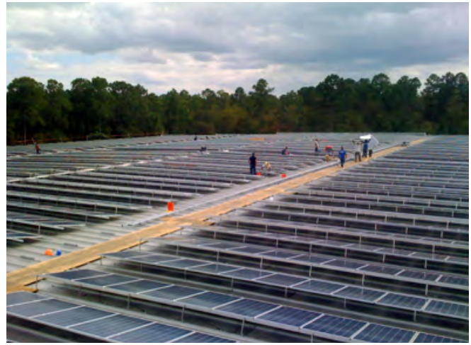
A 665-kilowatt third-party leased solar photovoltaic installation on a United Trucking warehouse. Photo: Sybac Solar.
