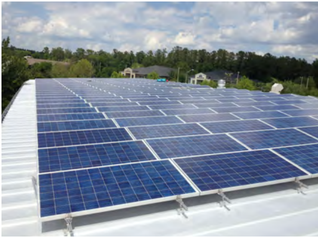
A 105-kilowatt solar photovoltaic installation on a leased commercial property. Photo: Solar Impact.
