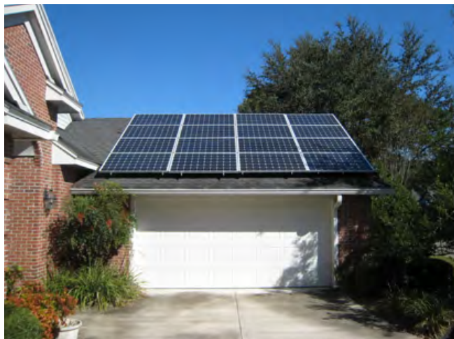
A residential 15-kilowatt solar installation using both net metering and feed-in tariff. (The two systems are not connected.) Photo: John Sheehy.
