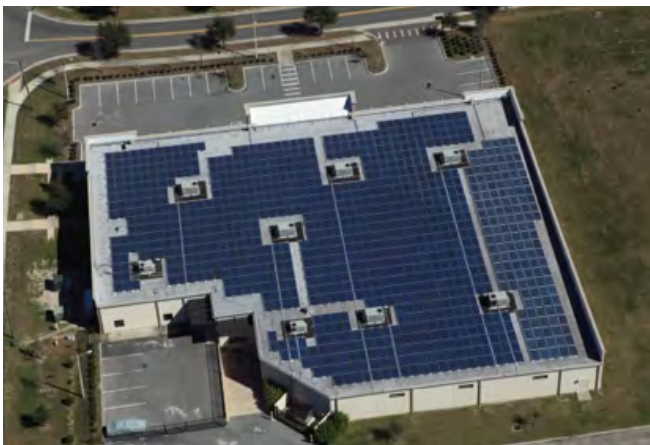
A 2-megawatt commercial solar installation undertaken as part of the Solar Feed-in Tariff program; the system was completed in two phases, from 2009 to 2010. Photo: Sybac Solar.
