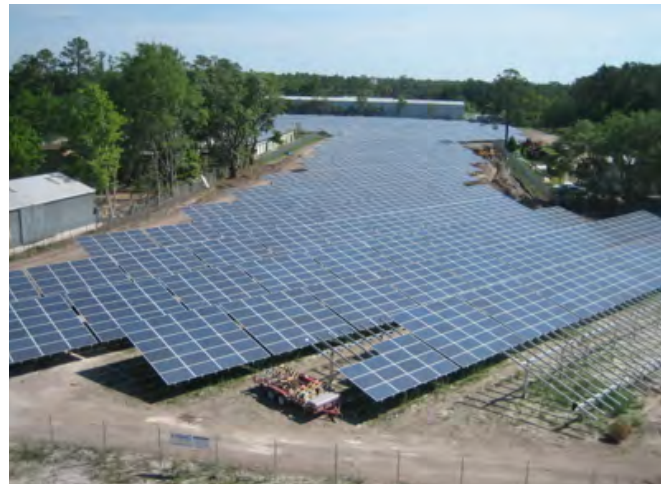
A 2-megawatt (MW) installation at 6th Street Solar Park. The two systems (a 1 MW fixed-panel system and a 1 MW single-axis tracking system) were completed in two phases, from 2011 to 2012. Photo: Sybac Solar.
