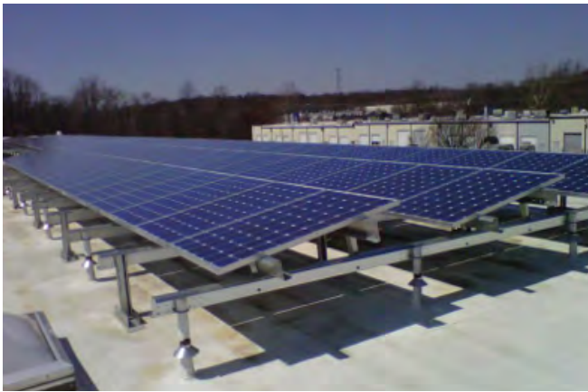
Solar photovoltaic panels at the Consolidated Warehouse and Fleet Maintenance Facility. Photo: Office of Central Services, Prince George's County.
