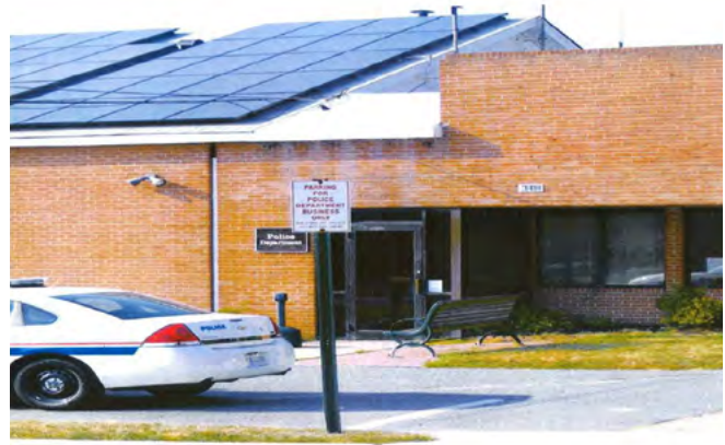
Solar panels on the roof of the Bladensburg Municipal Building.
