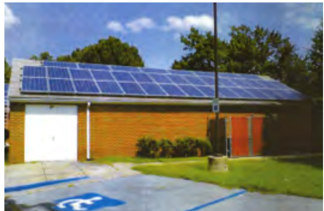
Solar Panels on the roof of Cottage City Government Office Building
