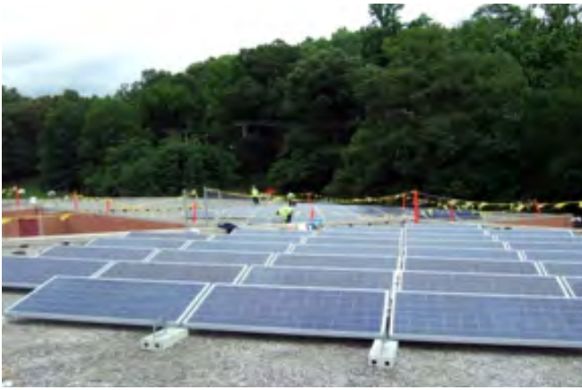
Rooftop solar photovoltaic panels at University Park Elementary School. Photo: Ross Salawitch.
