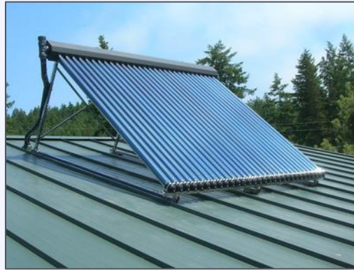
Solar Hot Water
