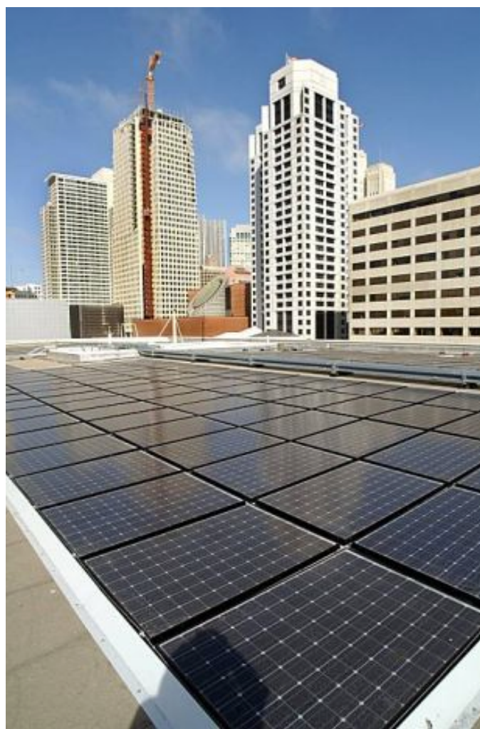
Solar panels on San Francisco's Moscone Center
