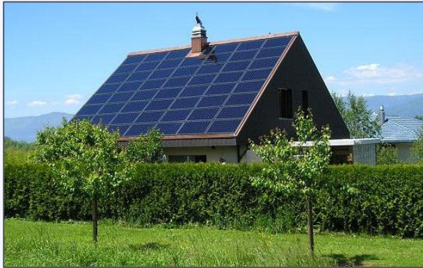
Solar Photovoltaic (PV)
