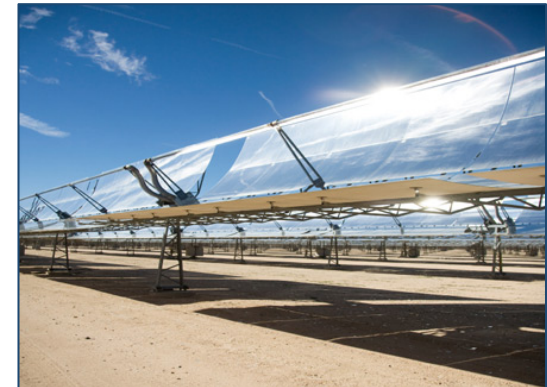
Concentrated Solar Power
