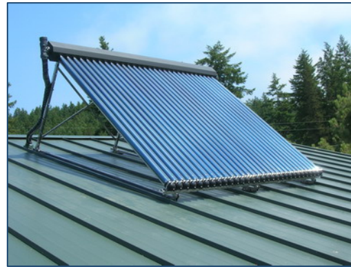
Solar Hot Water
