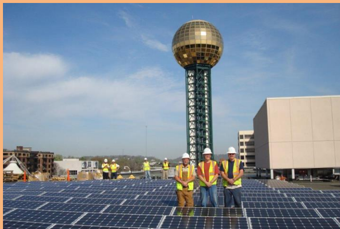
Knoxville Convention Center Solar PV Array (Photo Credit: International Brotherhood of Electrical Workers Local 790)
