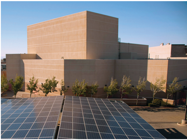
Solar array at Lancaster's Performing Arts Center.
