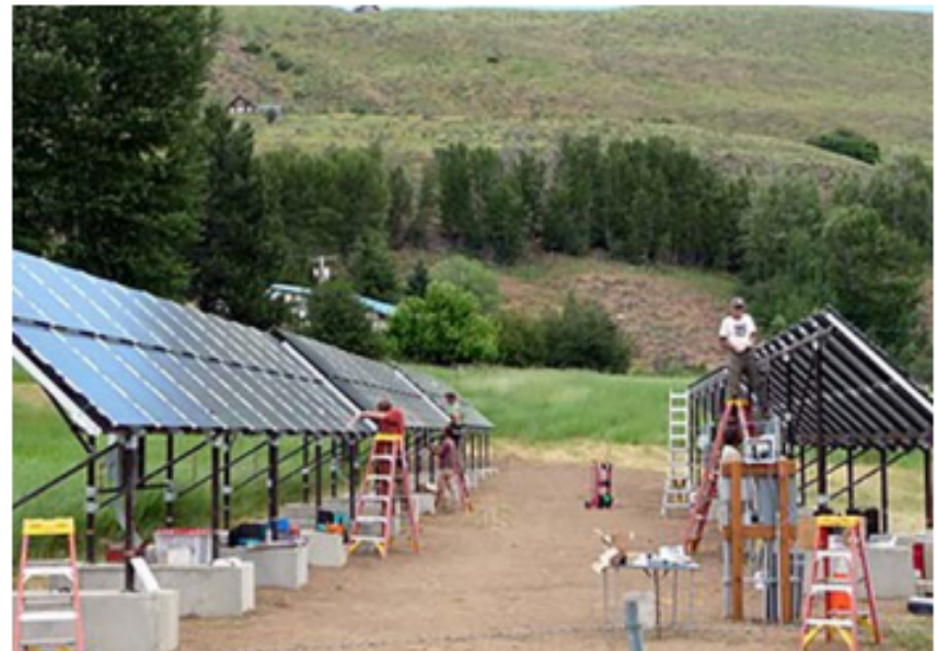
Winthrop Community Solar Project. Photo by Ellen Lamiman, Energy Solutions
