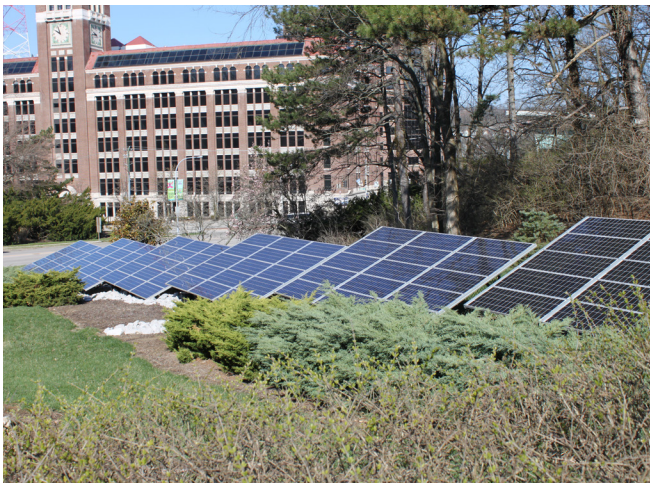
Ground mount system at the City's Parks and Recreation building.
