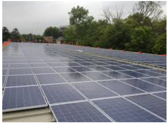
Array on the College Hill Recreation Center
