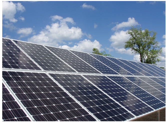
High-efficiency PV panels at WWTP
