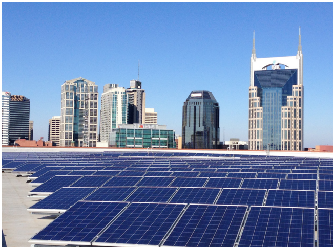
Solar Array on MCC
