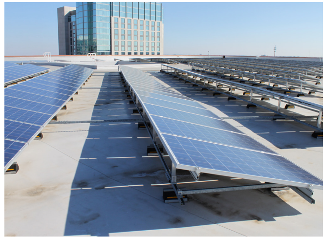
Panels on the MCC demonstrate inter-row spacing
