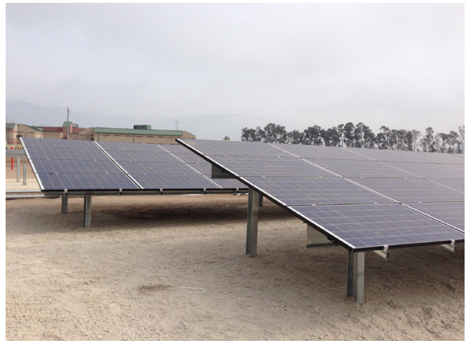
Completed solar installation at Todd Road Jail.
