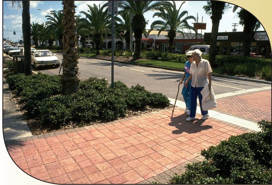
Crosswalk in Venice, Florida. Although attractive, the use of brick or pavers in crosswalks requires regular maintenance to maintain a smooth surface.
