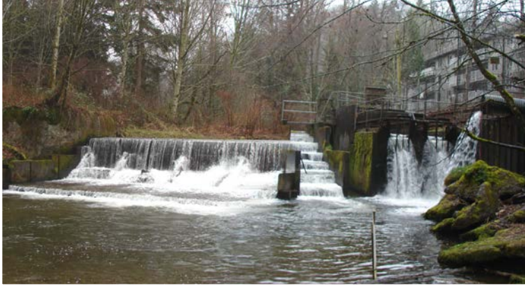
Hatchery Water Supply Intake Dam
