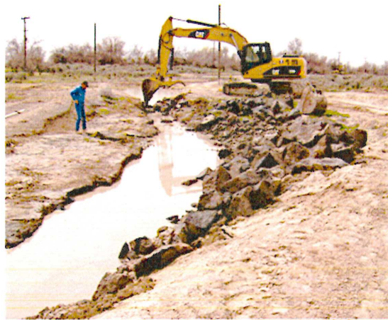
City crews begin developing new settling ponds to divert TSS from the canal system.
