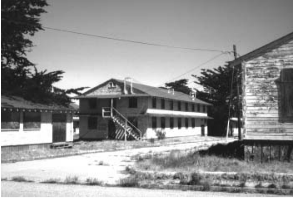
Army barracks with peeling LBP at the former Ft. Ord in Monterey, California
