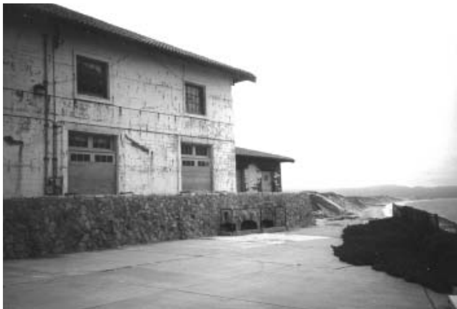
Deteriorating coastal facilities at the former Ft. Ord in Monterey, California
