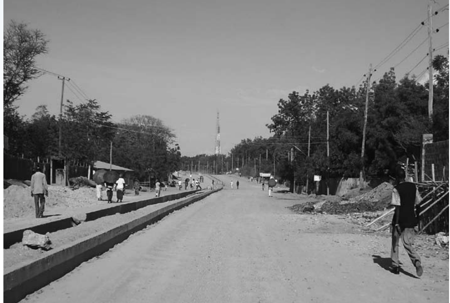
The government of the Gambella region is undertaking an ambitious project to pave streets in the main corridor of the city of Gambella as part of a sound, multimodal public transit system in that city.
